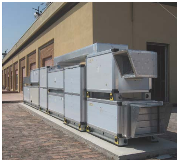
Figure 7.13 Photo of DEC air handling unit [13] and [32].
