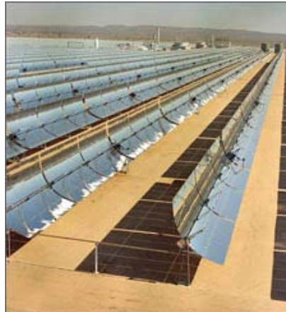
Figure 3.11 Luz solar power station for electricity production, southern California [3].
