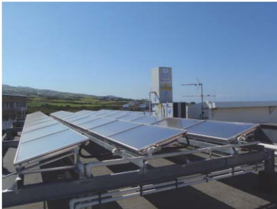
Figure 7.10 Solar collectors installation on the flat roof of the University of Reunion Island main building [13], [30] and [31].
