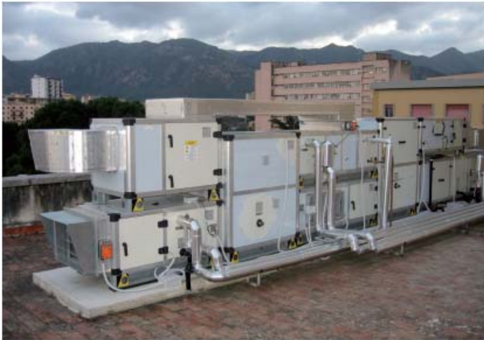
Figure 7.3 Desiccant air-handling unit equipped with heat pump (cools supply and heat up return regenerating air ) and two additional heat exchanger coils (nominal air flow 1500 m 3 /h), Dep. Energy, University of Palermo, Italy [13] and [25].
