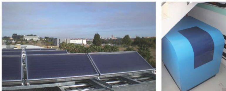
Figure 7.6 Double-glazed flat plate collectors field and adsorption chiller, laboratory/office building in Perpignan, France [13] and [27].
