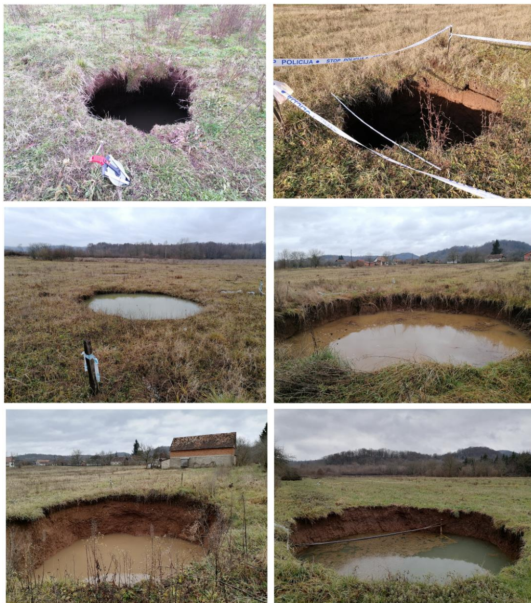
Figure 3. Photographs of several cover-collapse sinkholes that appeared after the Petrinja earthquake. The diameters of the sinkholes range from 1 to 10 m, with the exception of the main one (Figure 4).
