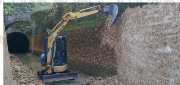
Figure 2: Removal of the tufa formed on the lateral sides of tunnel (URL 1).
