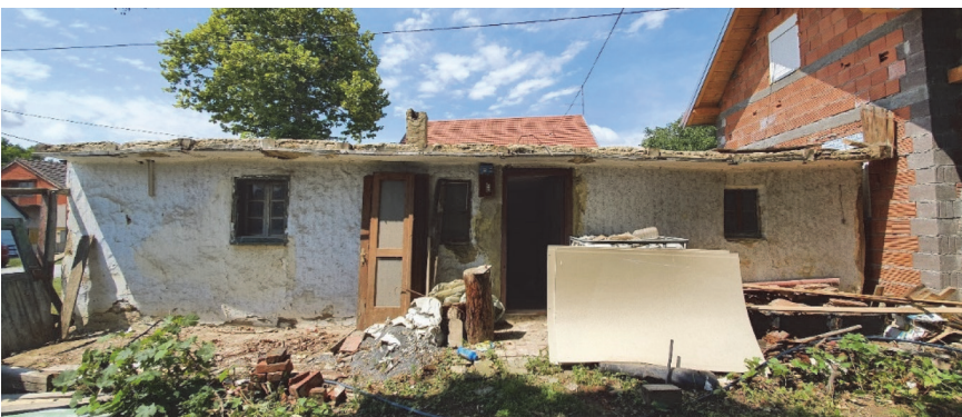
Figure 1. Ground floor of an earth house in Dopsin, shortly before the demolition (taken: July 2020)
