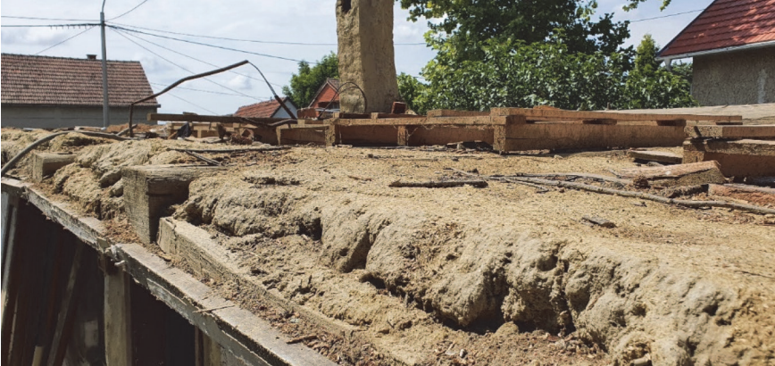
Figure 2. Floor structure of an earth house in Dopsin, shortly before the demolition (taken: July 2020)
