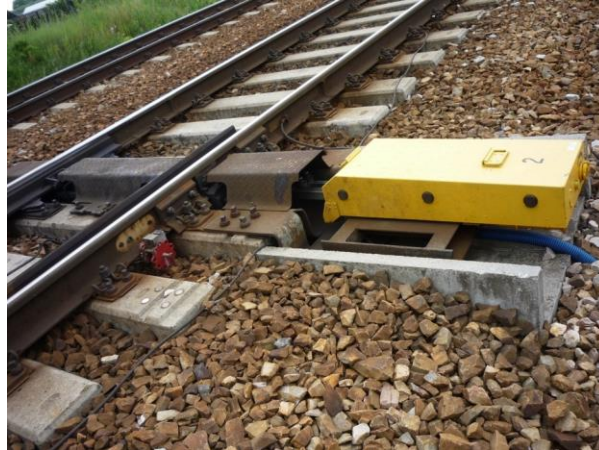
Figure 1: The switch motor used on national and international railway lines
