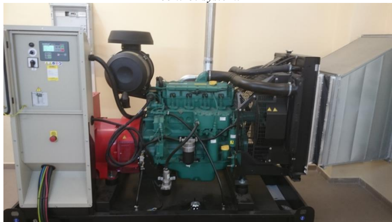
Figure 2: Power generator and controllers as an example of emergency power supply of railway traffic control system.
