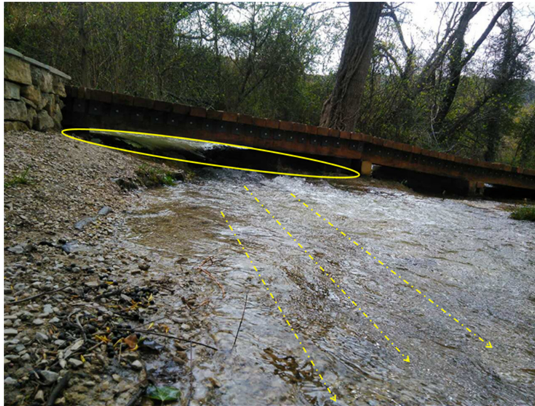
Figure 27. Water runoff below the path after removal of accumulated gravel.
