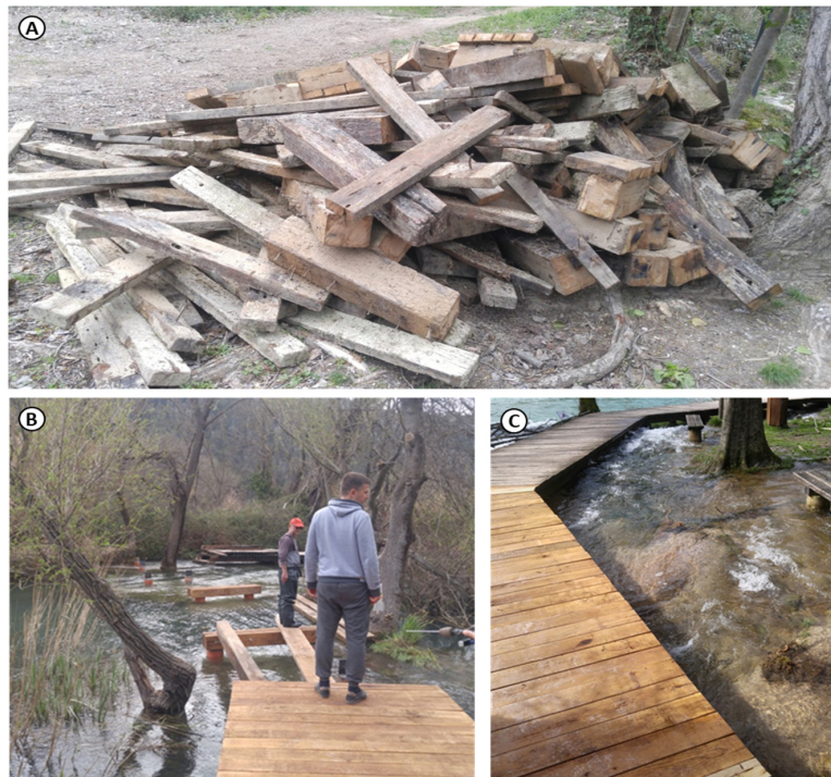
Figure 28. (A) Removed boards from the old path; (B) construction of the new path; (C) newly built path under which water runs unhindered.
