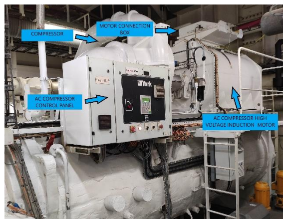
Figure 10: AC compressor unit
