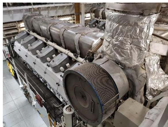
Figure 2: Diesel engine (prime mover)
