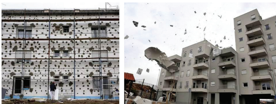
Fig. 3: Examples of low-quality construction work and its consequences.
