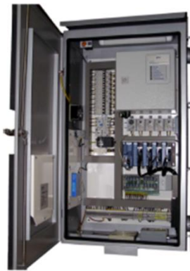
Information system cabinet
