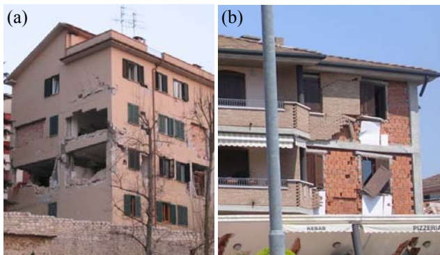
Figure 1. In-plane masonry infill/veneer damage and out-of-plane expulsion: (a) Abruzzo, Italy, 2009; (b) Emilia, Italy, 2012 (Magenes et al. 2012)
