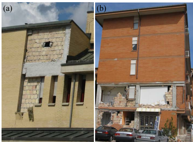
Figure 2. L'Aquila, Italy, 2009: (a) Out-of-plane masonry veneer expulsion; (b) Out-of-plane masonry veneer/infill expulsion
