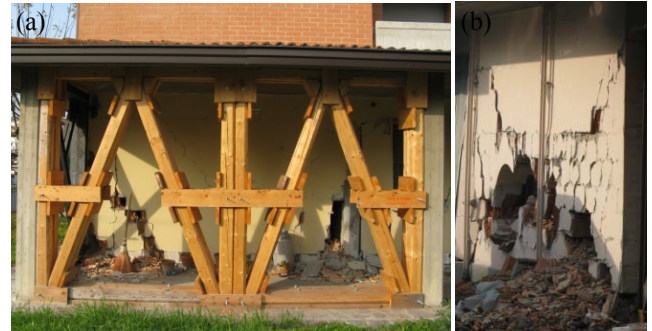
Figure 3. Emilia, Italy, 2012 (Manzini and Morandi 2012): (a) In-plane masonry infill damage and onset of out-of-plane expulsion; (b) In-plane masonry infill damage and out-of-plane expulsion
