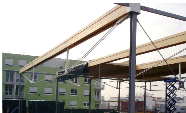
Figure 3. The installation of the roof hybrid construction of swimming pool in Sesvetski Kraljevac
