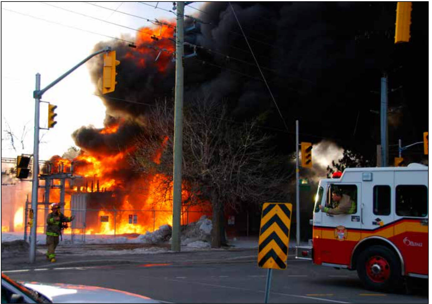
Substation power transformer on fire
