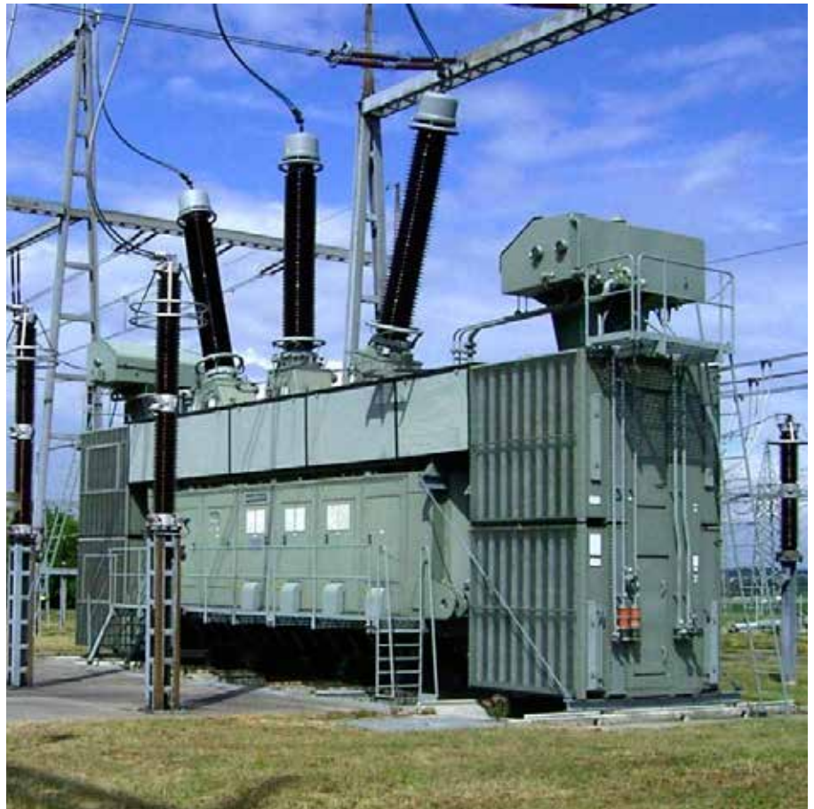
Healthy substation three phase power transformer
